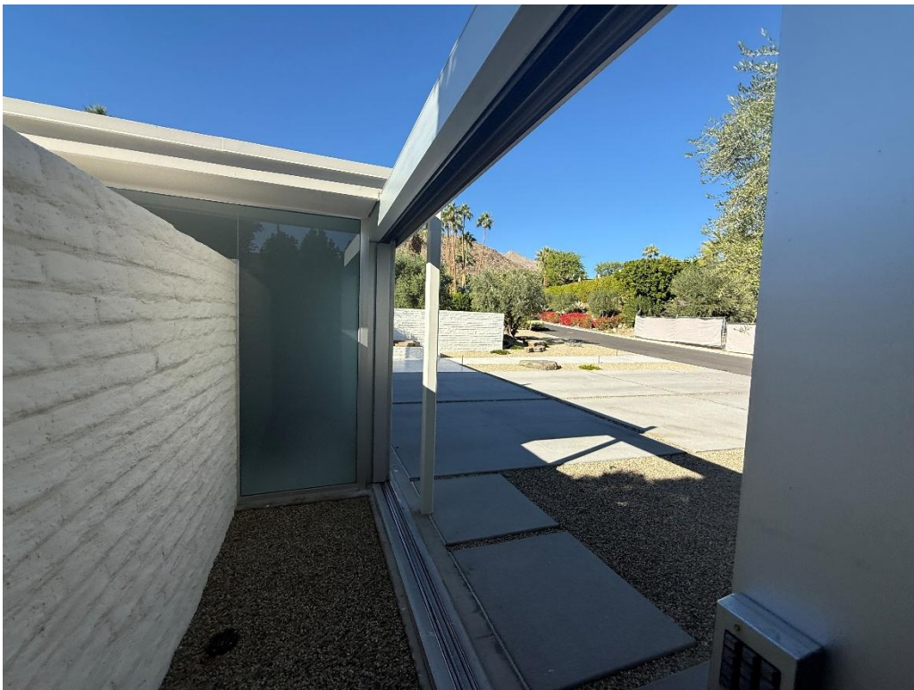
HVAC equipment and other systems in the corridor along the east façade. When the carport was enclosed and turned into a garage, the doors slide along this aluminum-clad spider leg detail.
