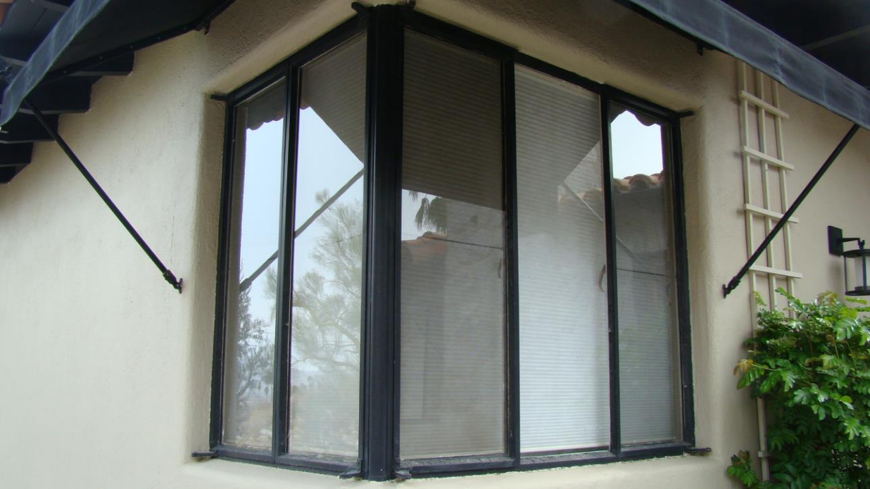
Metal Casement Window with Integral Pipe Support Located on the West Corner of Northwest Bedroom
