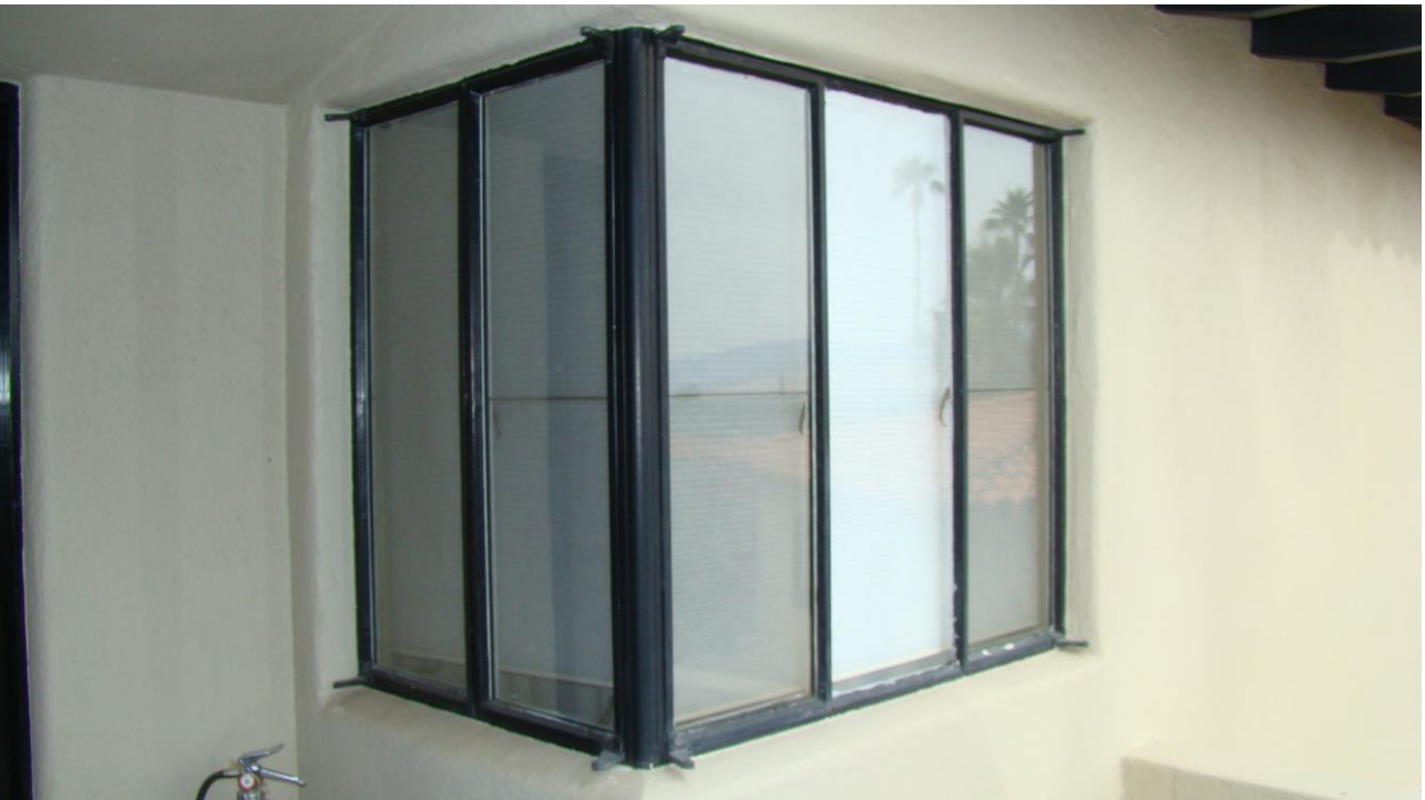
Metal Casement window with Integral Pipe Support Located on the SSE-Corner of ESE-Bedroom
