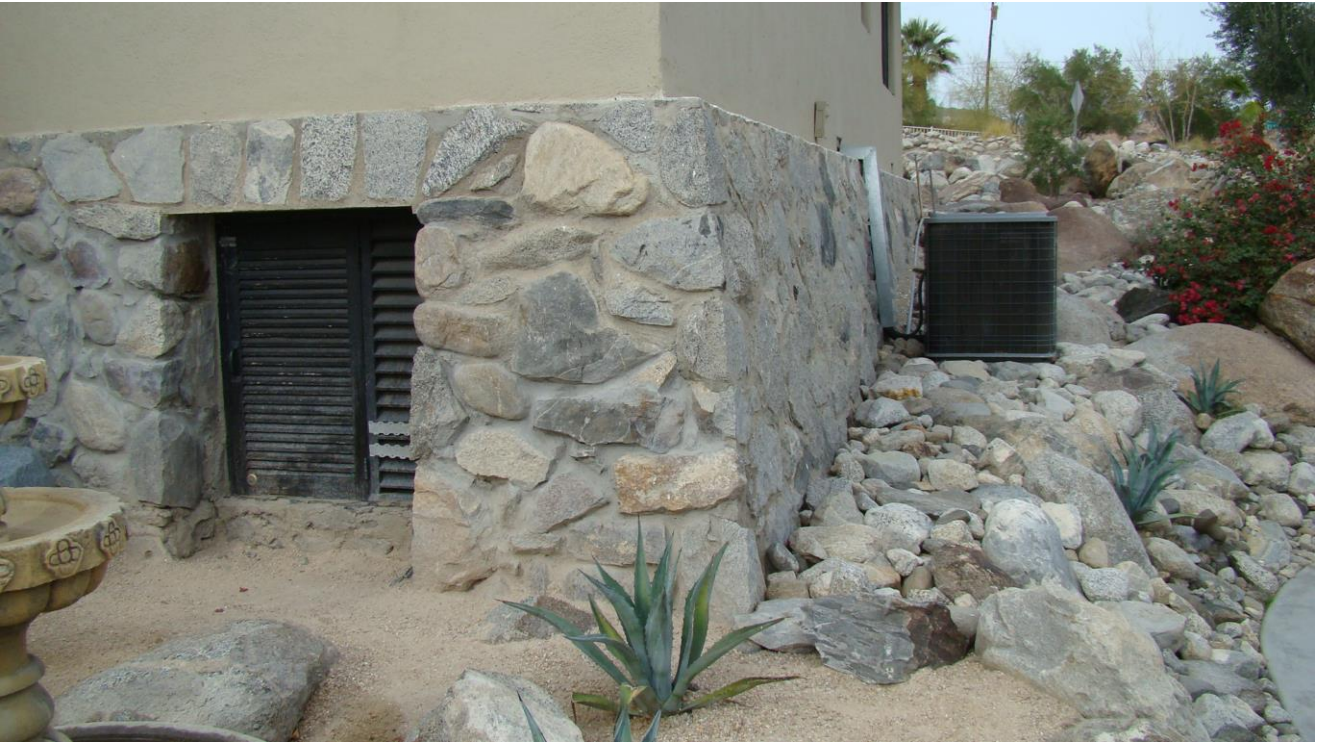
Stem Walls Form a 7-foot high Underfloor Area Entered Through an Access Door
