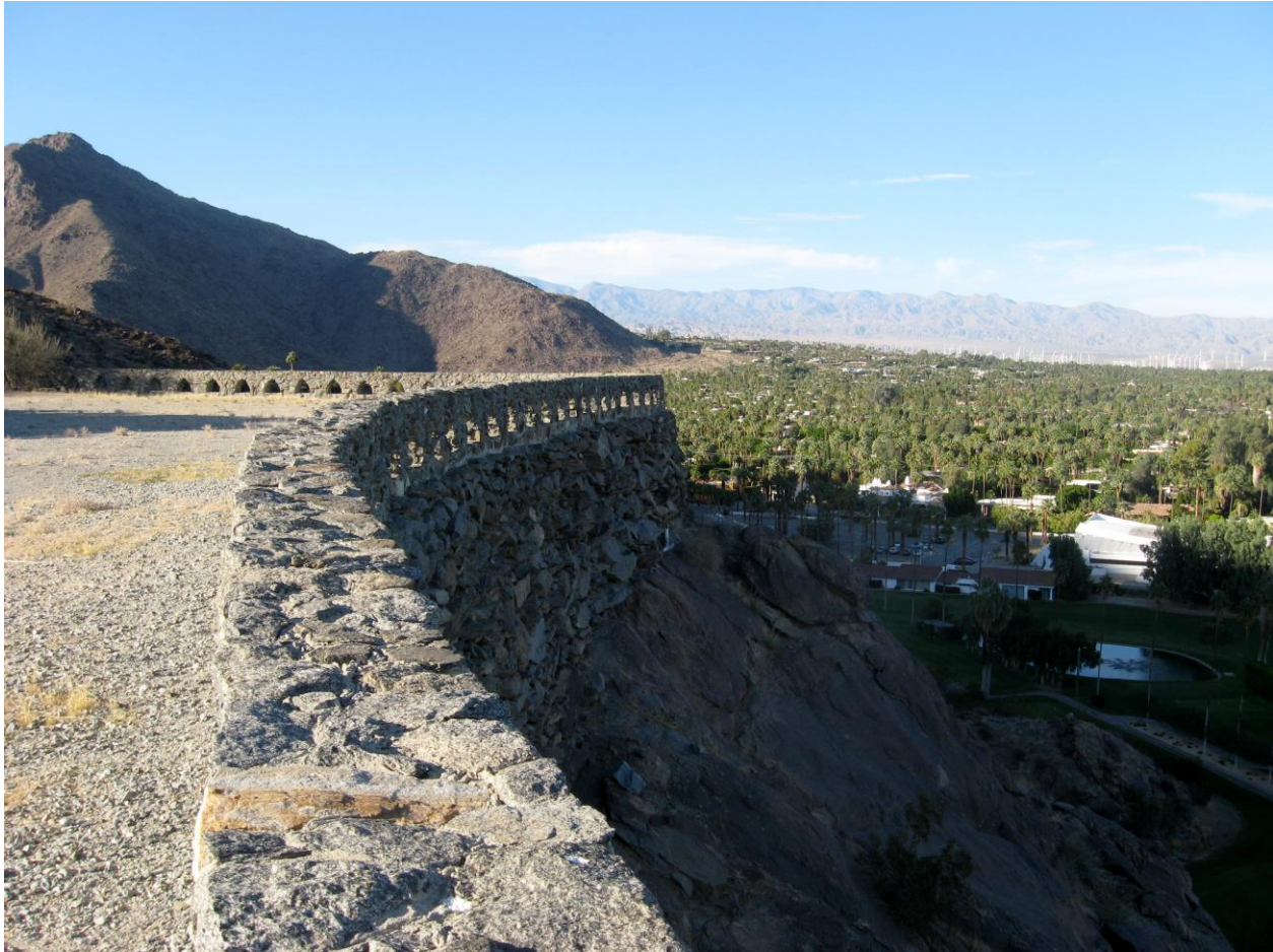
A view of Inspiration Point looking north towards Old Las Palmas showing stone retaining wall topped with perimeter wall incised with triangular openings.
