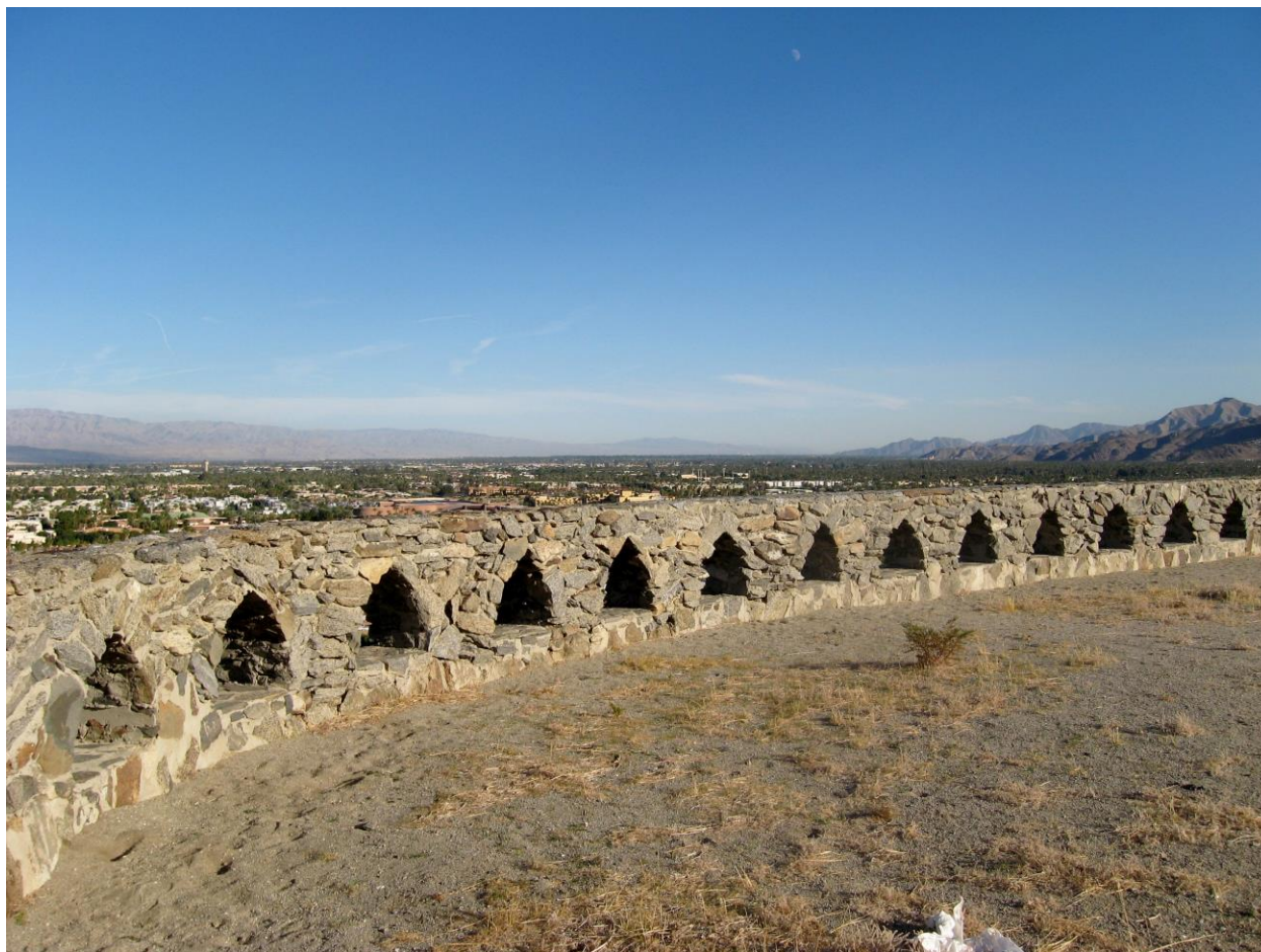
Detail of waist-high perimeter wall with triangular openings. View is to the southeast. (Author photo. November 2018)
