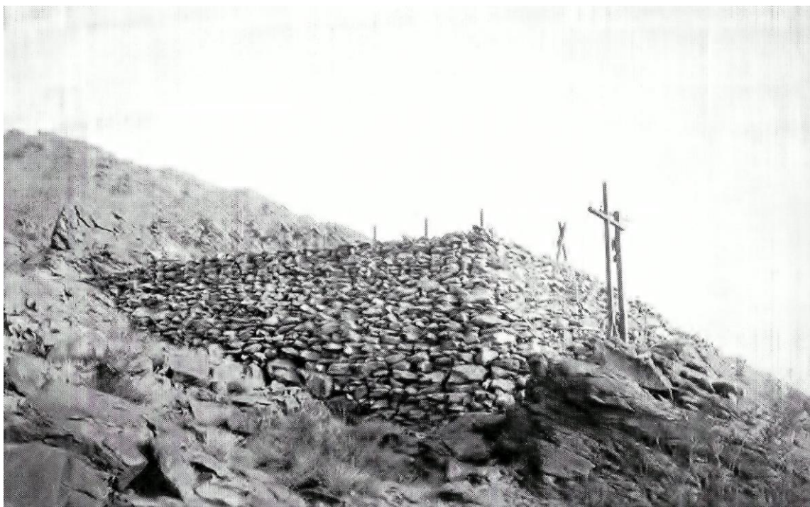
A view of the construction of the retaining wall for Ojo del Desierto. 1925. The technique and design would be repeated almost identically for the construction of Inspiration Point. (Courtesy Tracy Conrad)
